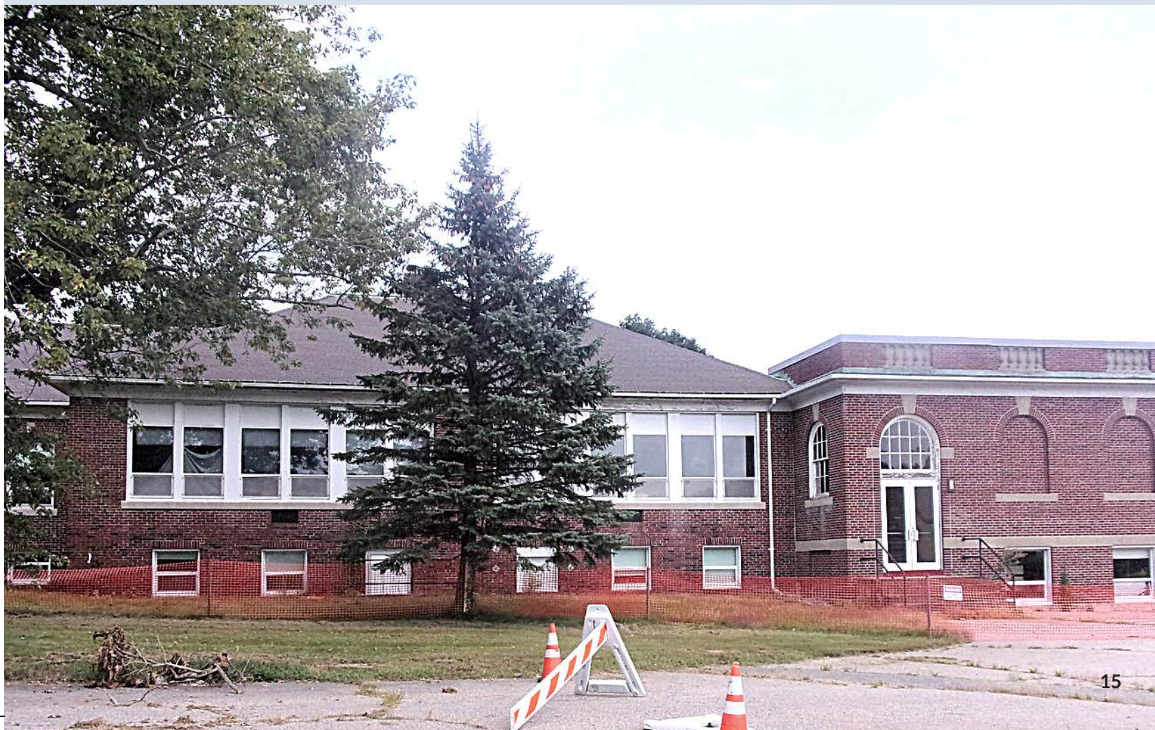
Anawan School in its deteriorated condition
